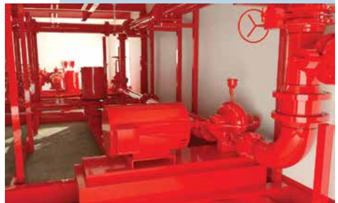
Interior Pump House Fire System
